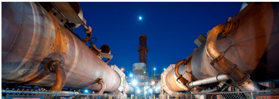
Rain CII Carbon calcined petroleum coke facility in Sulphur, La. Source: Rain CII
